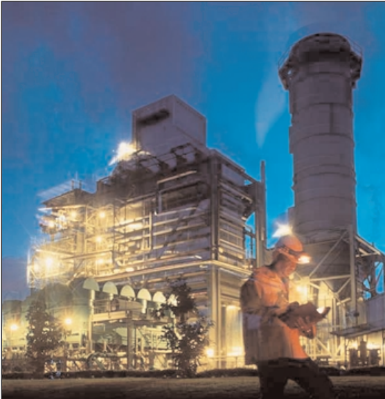
Combined Cycle Power Plant
