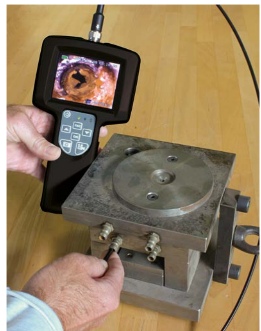
Fig.: Corrosion in the cooling duct
