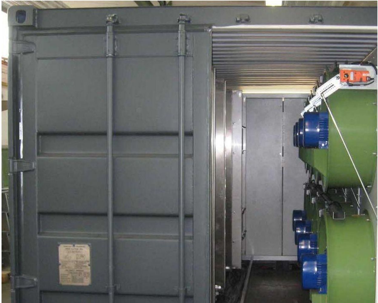
Cooling by fan
